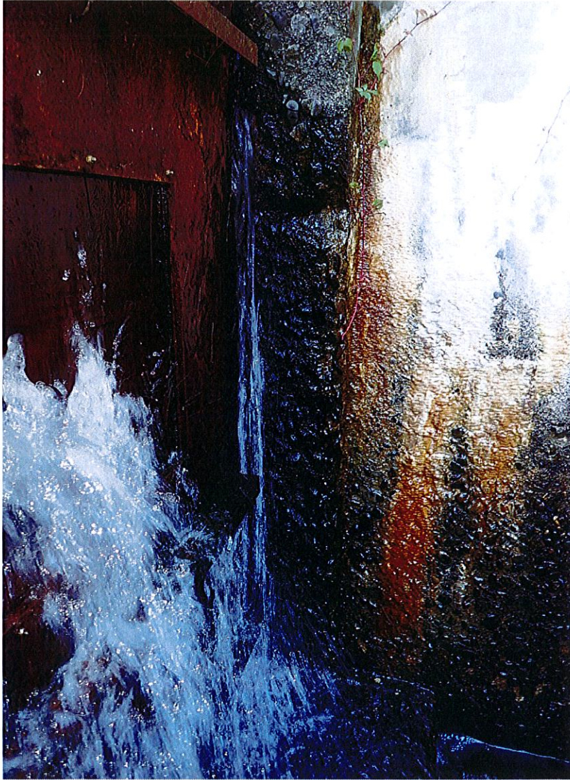
PHOTO 6 CONCRETE DETERIORATION ON GUIDE ON LEFT SIDE OF DAM
