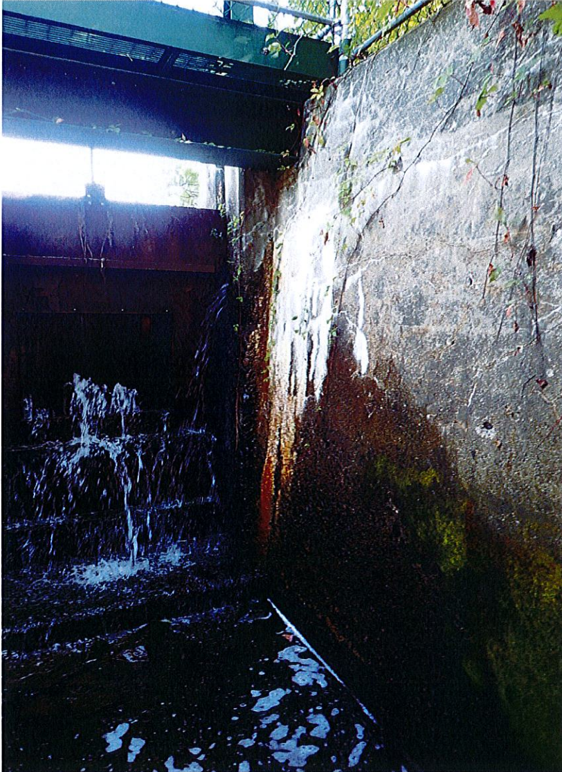
PHOTO 4 OVERALL CONCRETE DETERIORATION ON LEFT SIDE OF DAM
