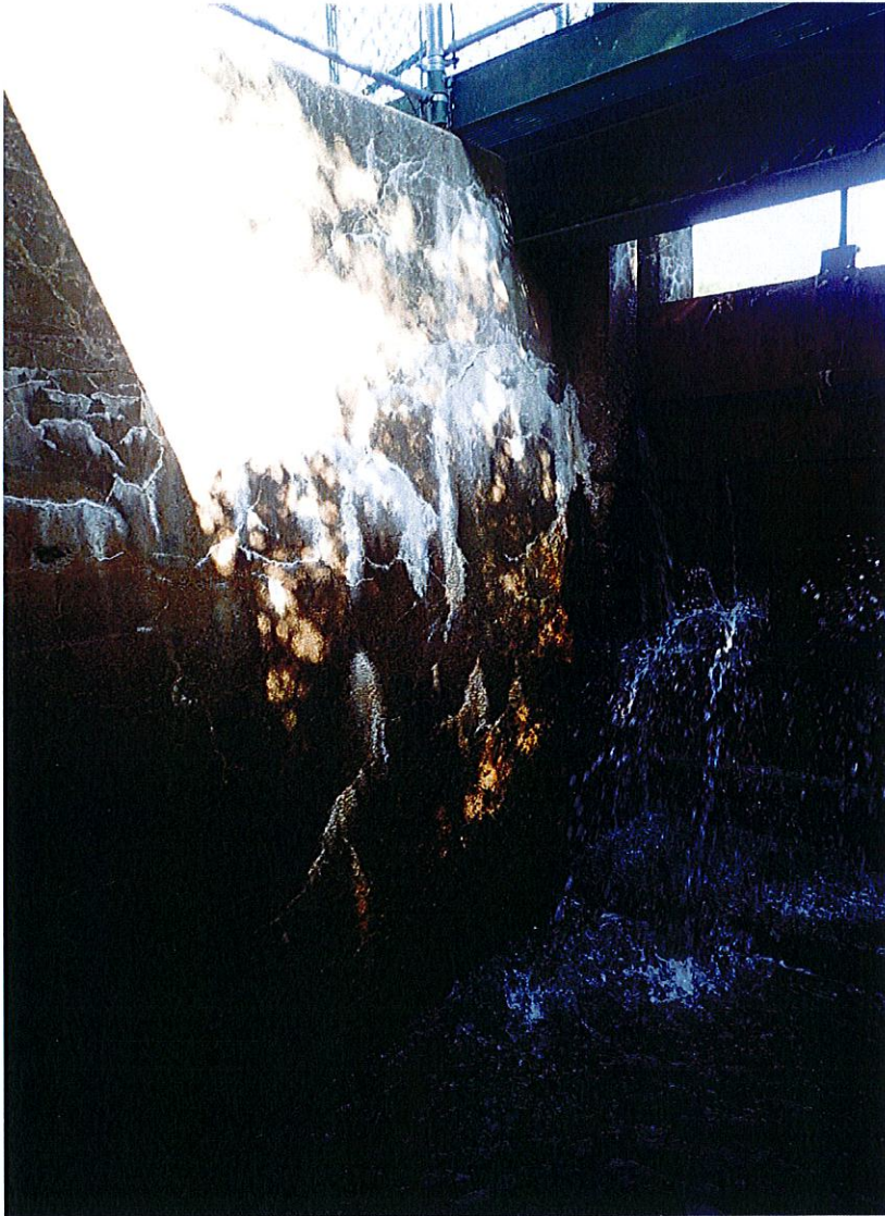
PHOTO 3 OVERALL CONCRETE DETERIORATION ON RIGHT SIDE OF DAM
