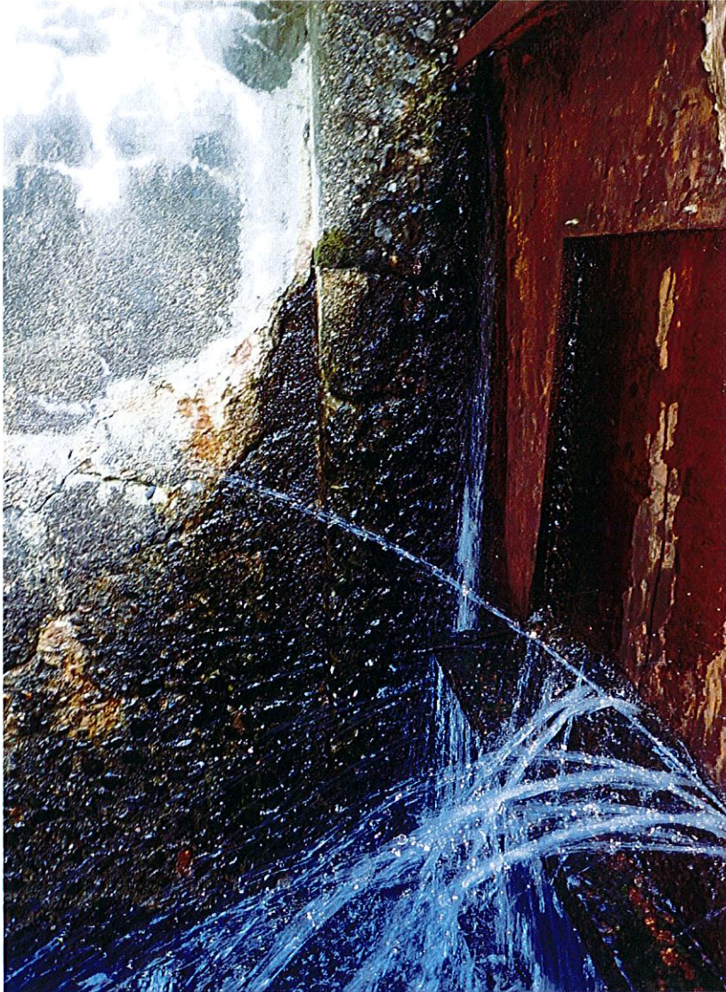
PHOTO 5 CONCRETE DETERIORATION ON GUIDE ON RIGHT SIDE OF DAM
