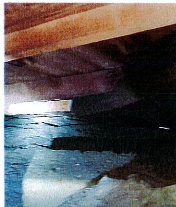
Hip rafter broken
