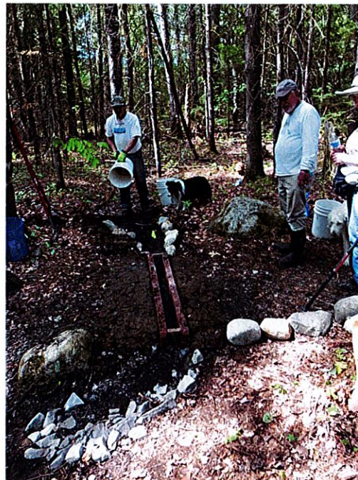
Commission members at work installing drain- age structures at Torsey Pond Nature Preserve
